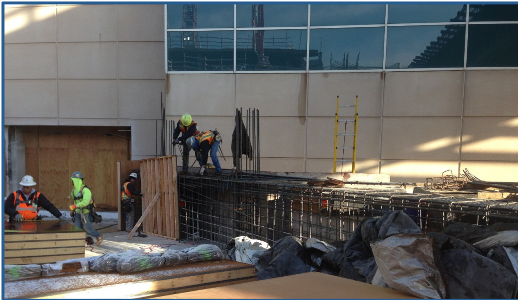
Figure 4: Right Sidewall at Level 3 Area F
