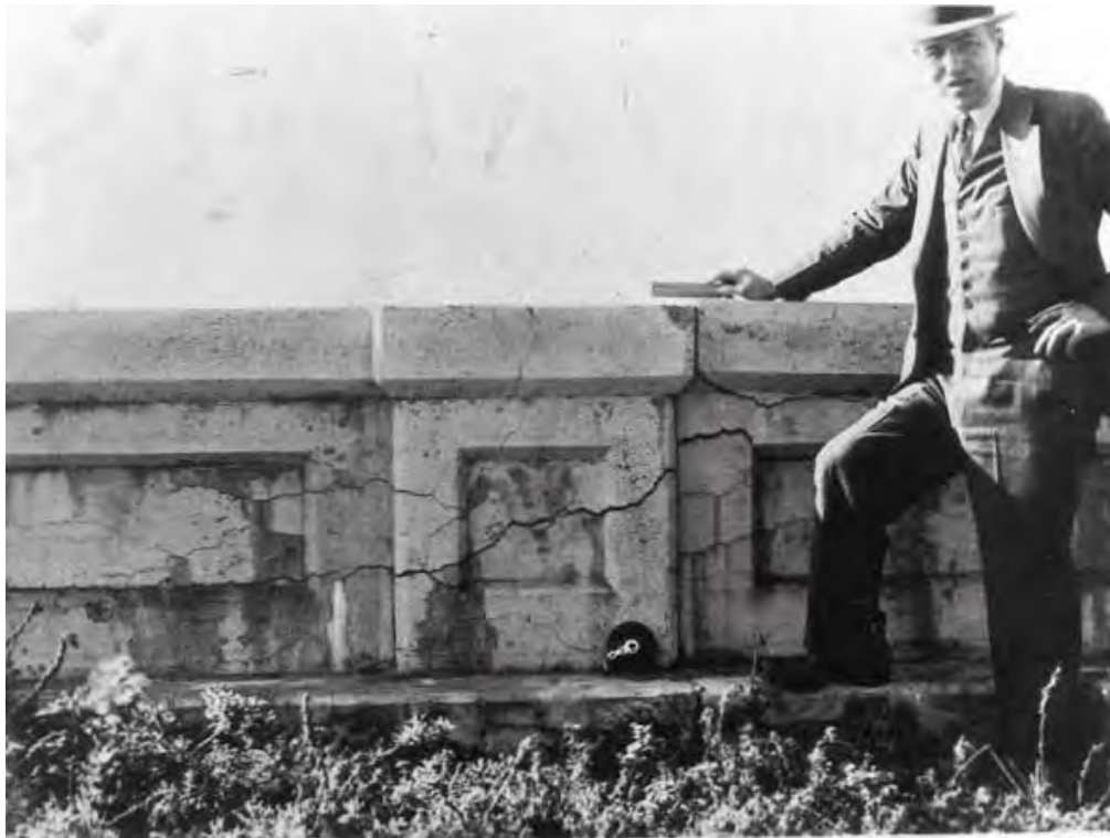
Figure 3.208. Thomas Stanton of the California State Division of Highways and a Bridge Parapet Wall that is Showing Signs of Damage due to Alkali-Silica Reaction From Alkali-Aggregate Reactivity (AAR) Fact Book ; (FHWA, 2013)
