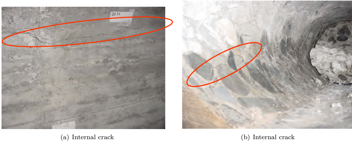
Figure 17.11: Observed internal crack
